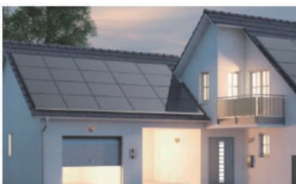
Household rooftop photovoltaic power station
