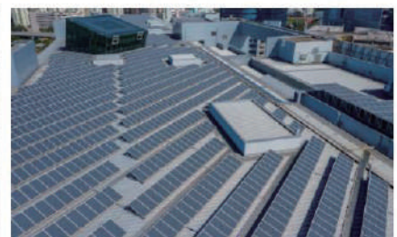
Industrial and commercial park building rooftop photovoltaic power station
